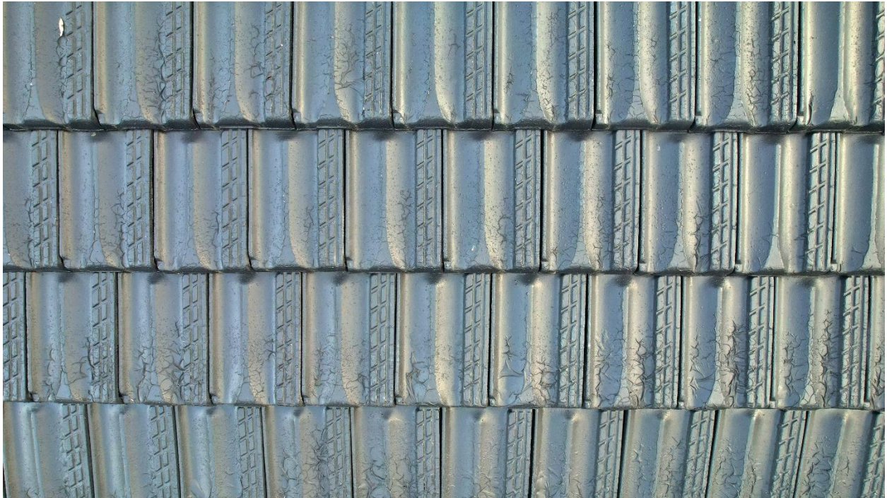
Photo 2 – Close up of roof section, showing peeling and cracking
