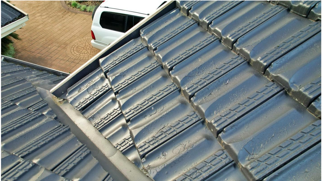
Photo 2 – Close up of bubbling and cracking can be seen
