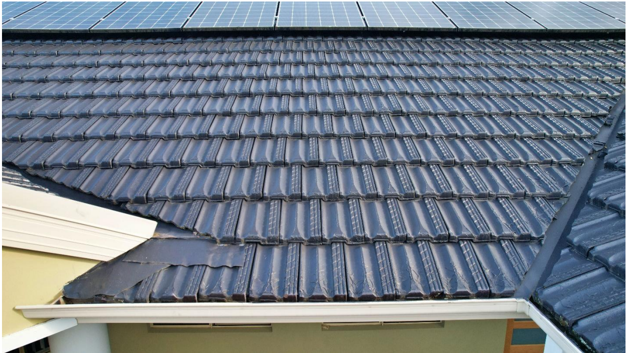
Photo 4 – Close up of roof section along the gutter line, showing peeling, bubbling and cracking paint which extends from the gutter to solar panels
