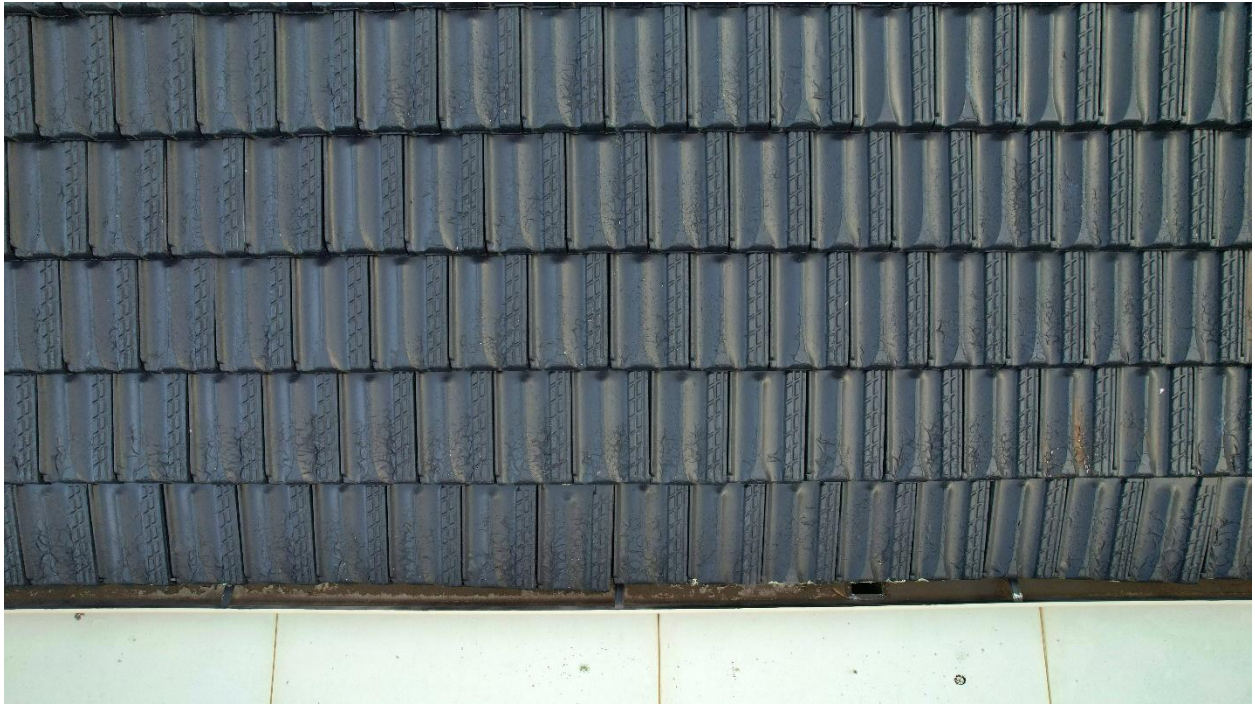
Photo 3 – Close up of roof section, showing peeling and cracking
