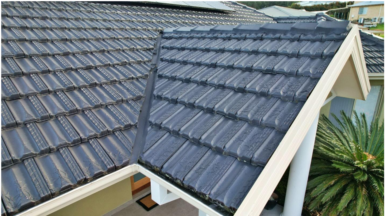
Photo 5 - Close up of roof section along the gutter line, showing peeling, bubbling and cracking paint
