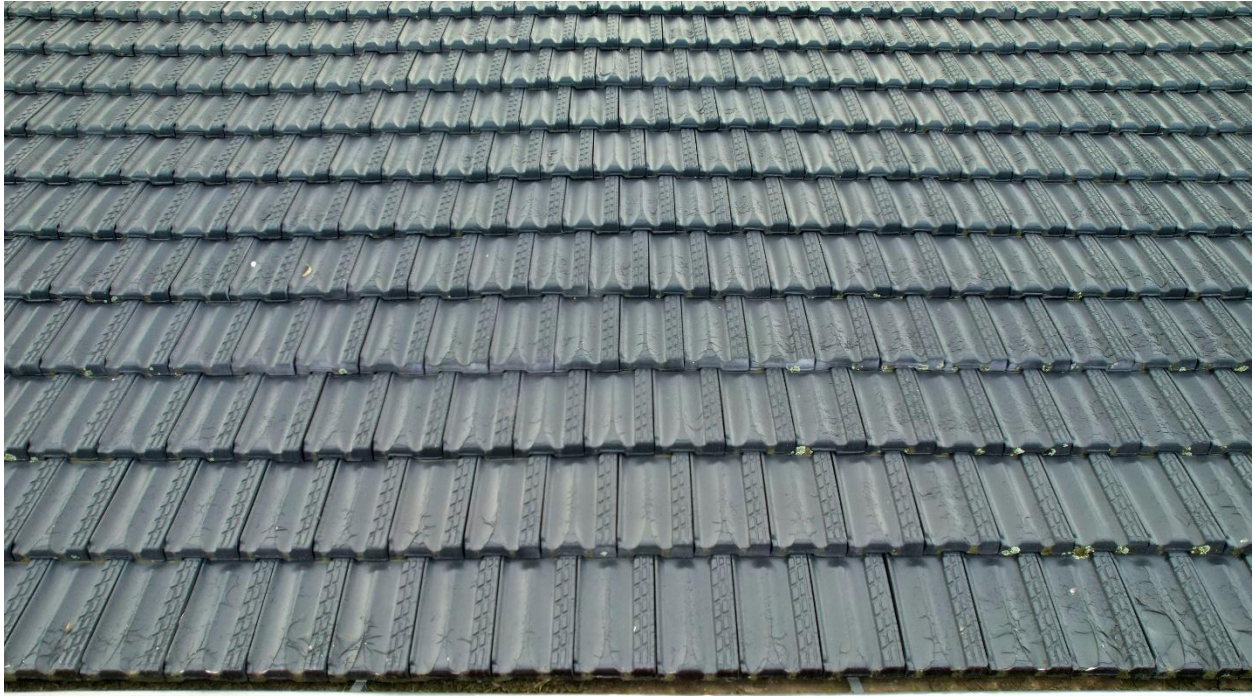
Photo 6 - Close up of roof section along the gutter line, showing peeling, bubbling and cracking paint
