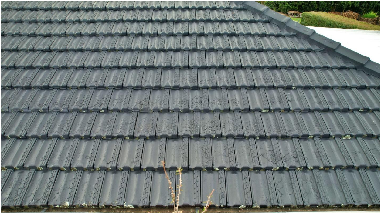
Photo 7 - Close up of roof section along the gutter line, showing peeling, bubbling and cracking paint
