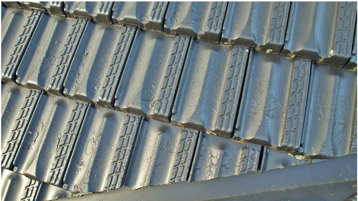
Photo 3 – Close up of bubbling and cracking can be seen
